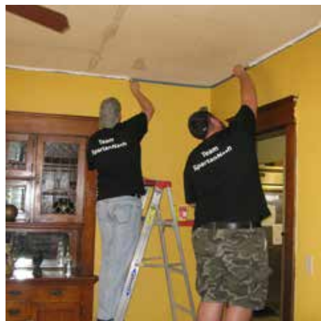
Volunteers from Nash Finch give the dining room at our shelter a fresh coat of paint as part of their annual Helping Hands day.
